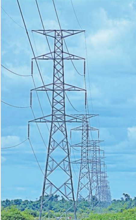
230 KV Transmission line, LAOS
